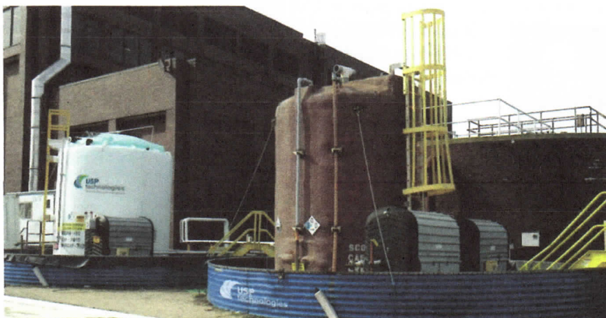
The Bergen Point Wastewater Treatment Plant (Babylon, N.Y.) has experienced notable cost savings after installing USP Technologies (Atlanta) PRI-TECH® technology, which includes a hydrogen peroxide system (left) and ferrous chloride system (right). USP Technologies
